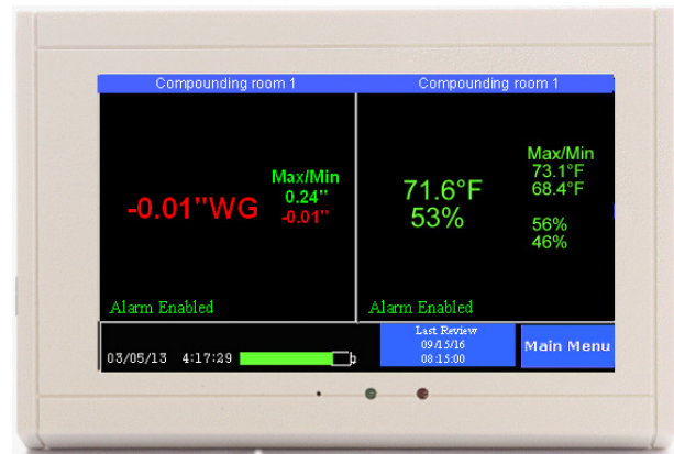
Red Alert on Unsafe Conditions
